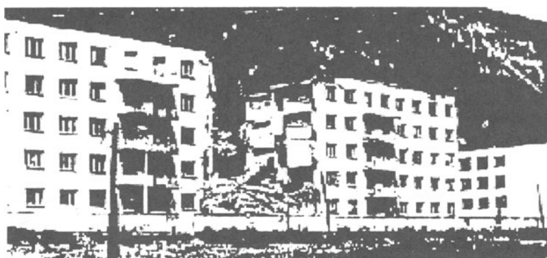
Figure 2. Racha earthquake (Georgia, 29.04.1991): a) general view and damages after main shock of hostel building of technical training college in Ambrolauri; b) collapse of middle part of a building after an after-shock (3.05.1991)
